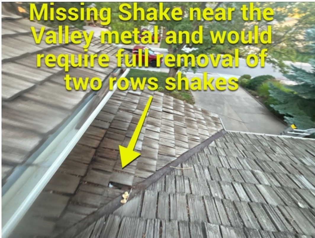
PHOTO 05 / MISSING SHAKE NEAR VALLEY
