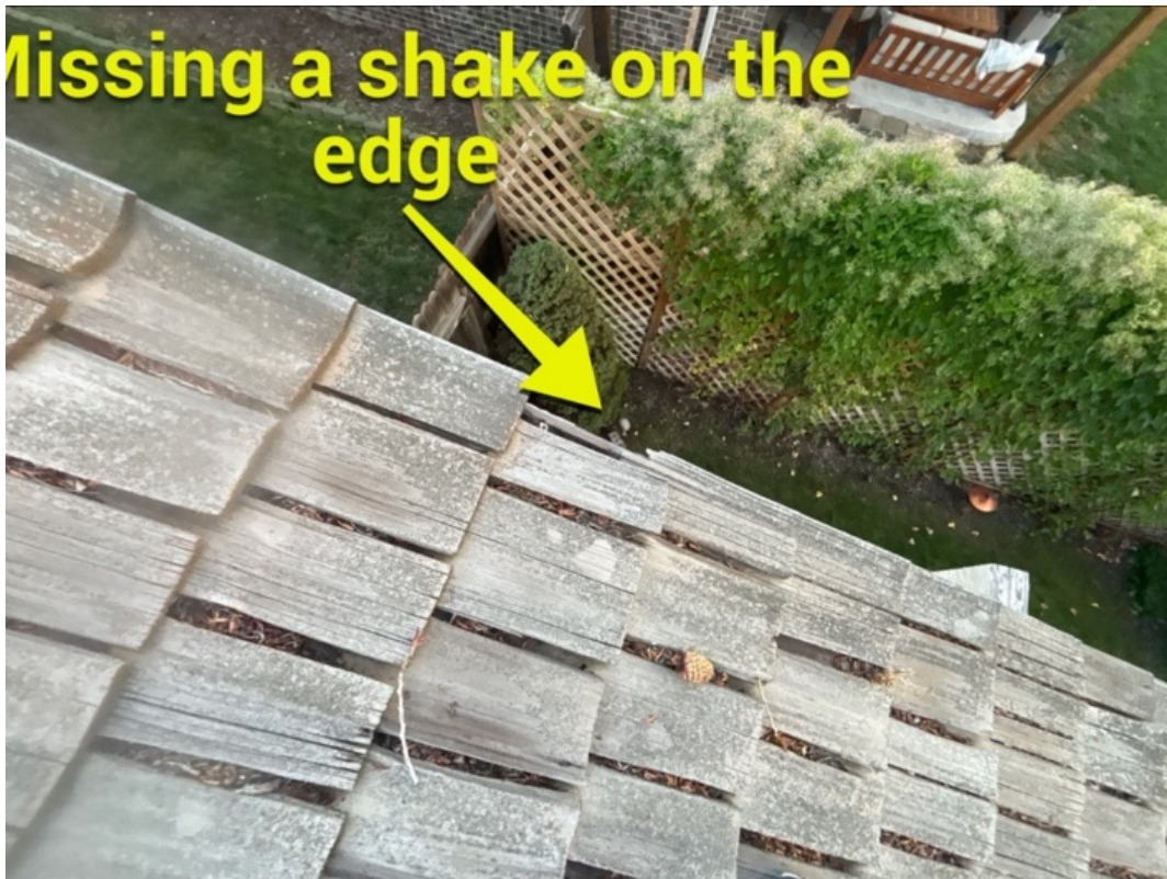
PHOTO 09 / MISSING EDGE PIECE
